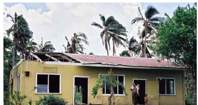
House on Upolu, Samoa which was damaged by Cyclone Heta in January 2004 (photo by Ilan Kelman).
