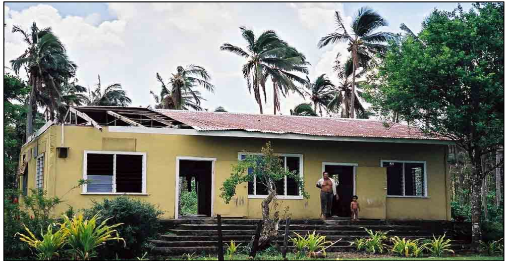
A house on Upolu, Samoa that was damaged by Cyclone Heta in January 2004. (Photo by Ilan Kelman)
