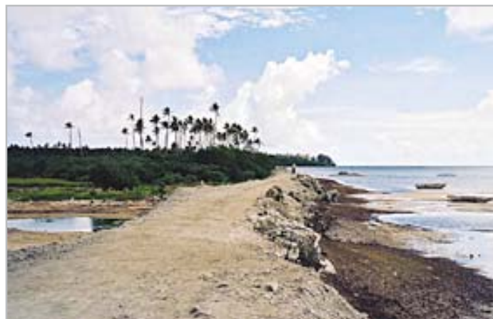
A seawall in Tonga Islands damaged from wave force impact. (Photo source: I. Kelman)
