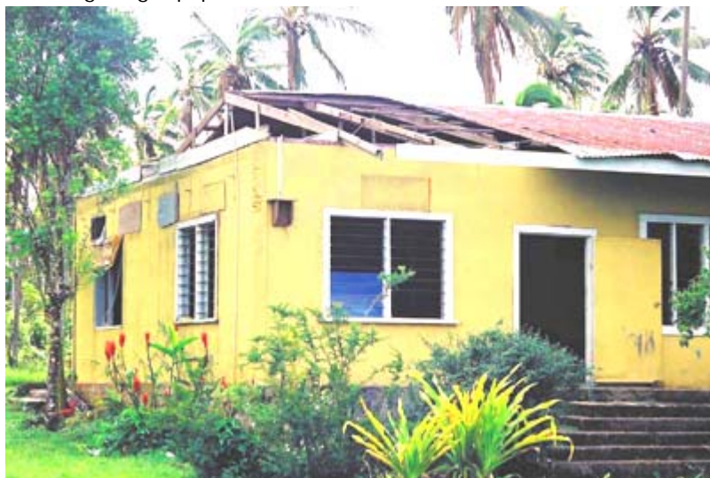
A house in Upolu, Samoa, damaged by Cyclone Heta in January 2004. Photos courtesy of Ilan Kelman
