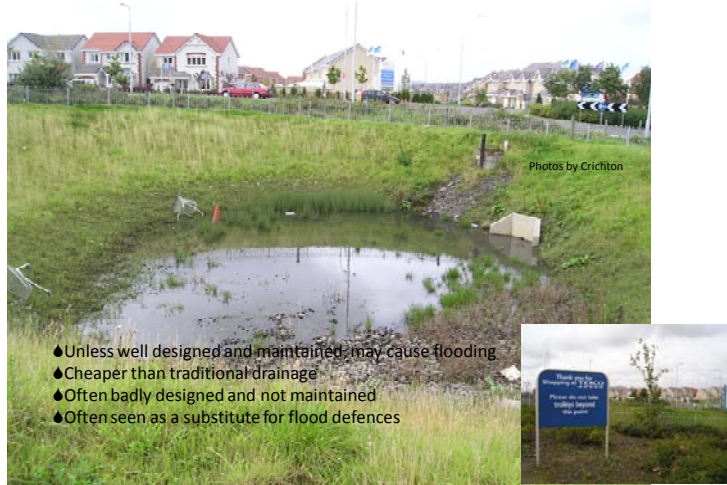
Sustainable drainage systems (SUDS) A SUDS pond complete with trolleys and rubbish.
